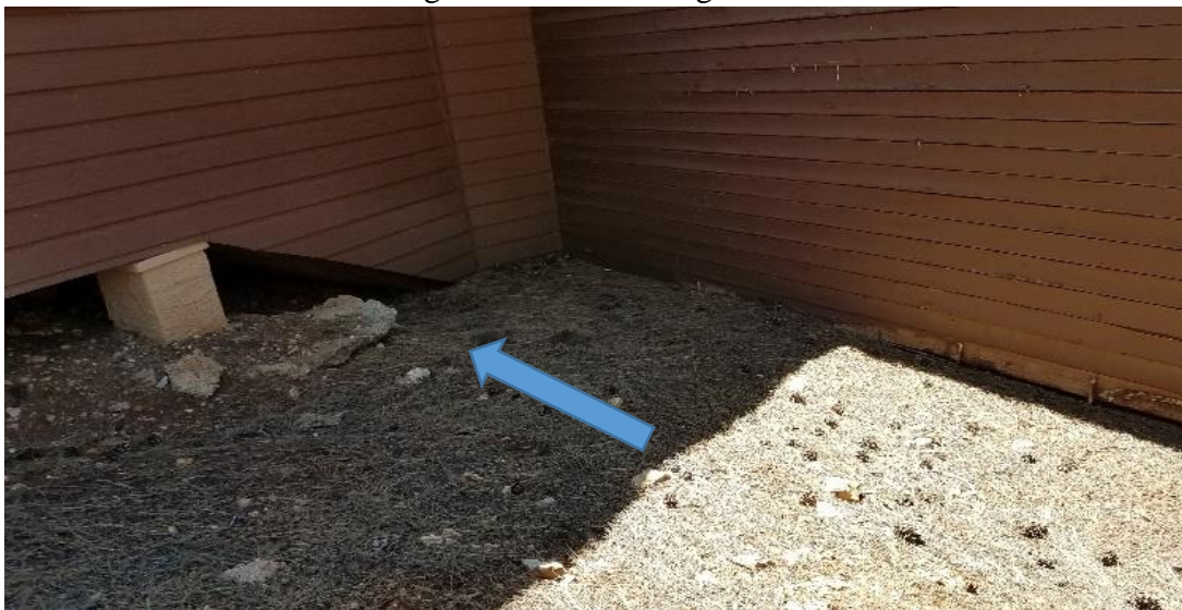
Figure 7: GCHS foundation A, problem area 4
