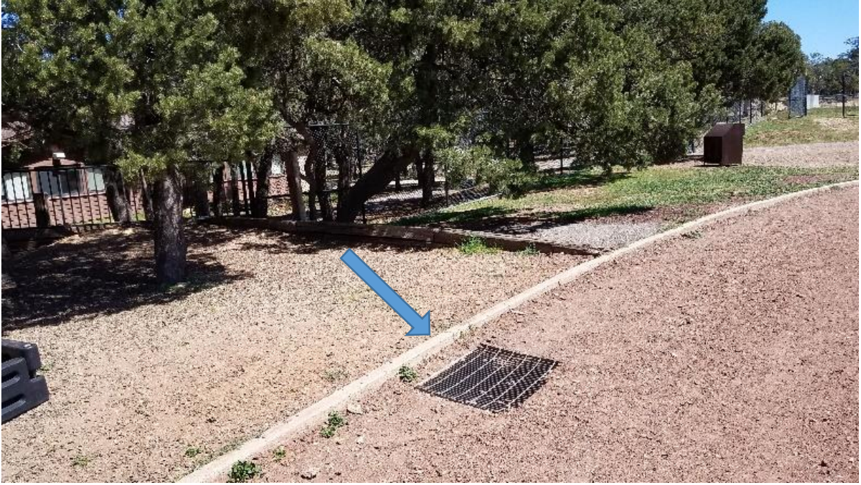
Figure 12: GCHS drainage tank / basin B, problem area 7
