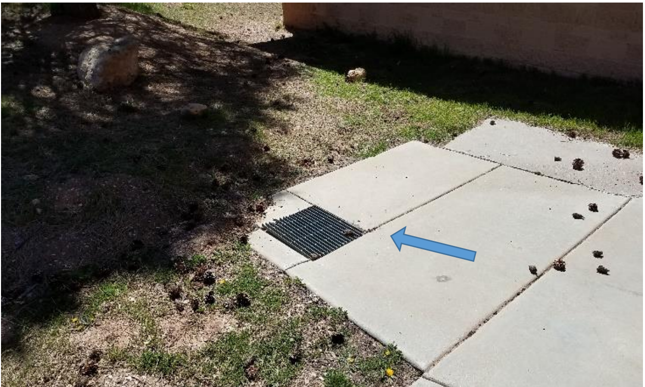
Figure 11: GCHS drainage tank / basin A, problem area 7
