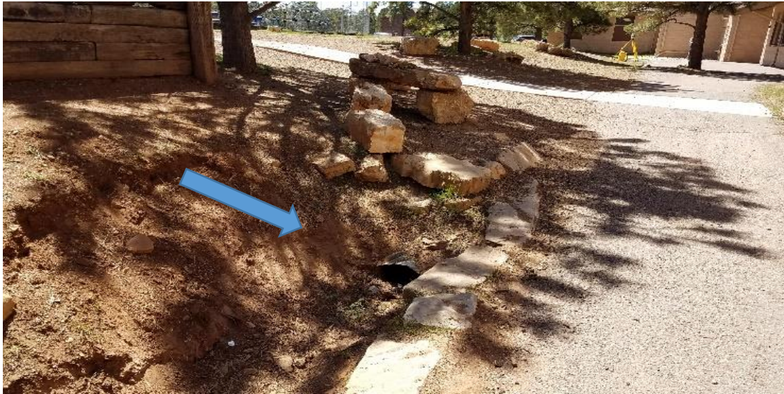
Figure 6: GCHS culvert B, problem area 3
